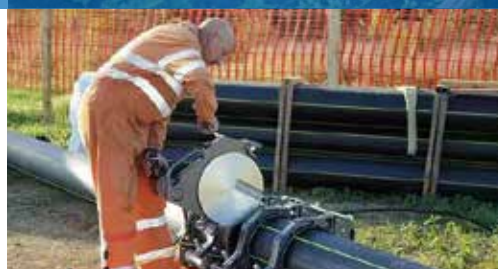
燃气管 Gas supply pipe
