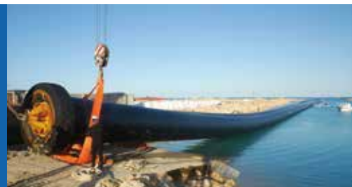
给水管 Drinking water supply pipe
